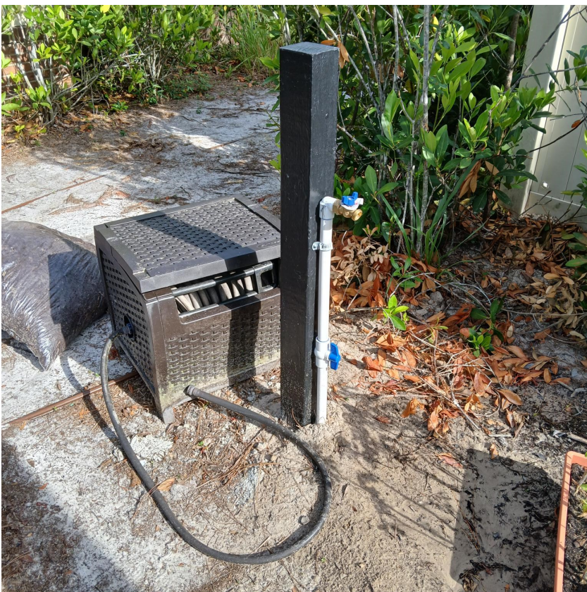
Water line and faucet installed for Garden club Added water line from the phase 2 pump room.
